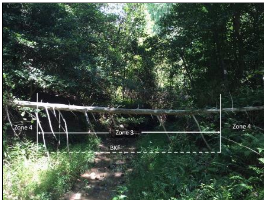
Figure 33. Example of bridge located in Zone 3 with intermediate structure (Upper Stick Elliott Creek – Cleveland County, NC).
